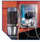
Barrier fluid, dosing pump
